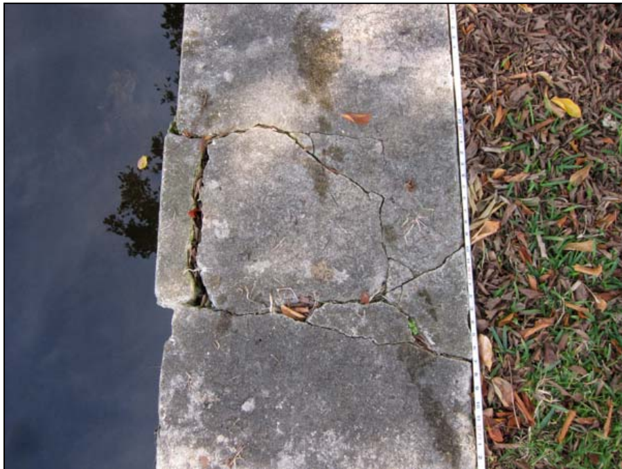
Photo 10: View of breakage with unsound concrete in the cap at Station 0+36.
