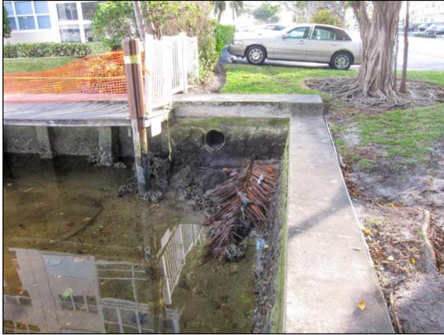
Photo 1: View of the Property bulkhead looking east at Station 0+00. Note depressions in upland soil and accumulation of sediment at toe of wall.
