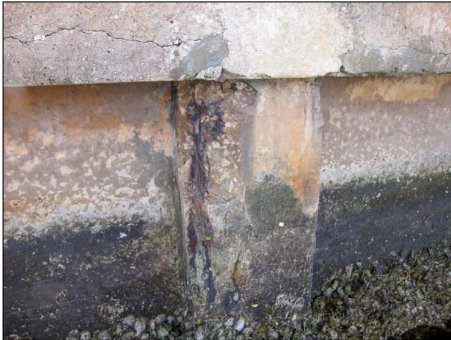
Photo 18: View of typical spalled and unsound concrete with exposed corroding internal steel in a T-pile. Note longitudinal cracking in the cap above.
