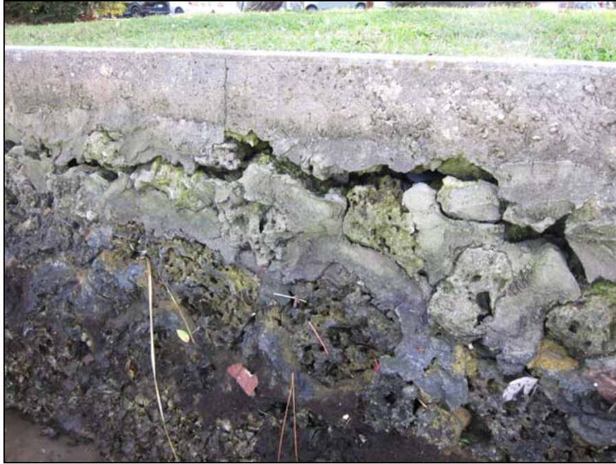
Photo 13: View of typical separation between the limestone rocks along the eastern portion of the Property bulkhead.
