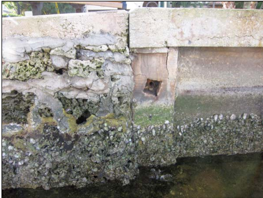
Photo 16: View of the transition from the limestone rock wall to the concrete pile/panel wall with an empty tie rod end connection recess in the T-pile. Note cracked and unsound concrete in the T-pile, as well.
