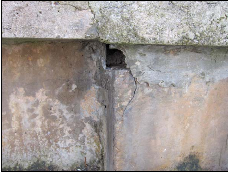
Photo 19: View of a gap between the top of a concrete T-pile and the cap above.
