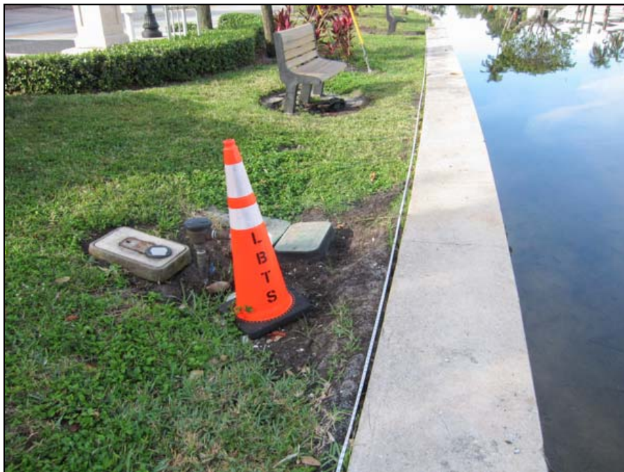
Photo 4: General view of the Property bulkhead with eroded soil behind the cap.
