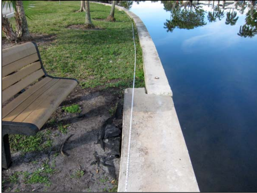
Photo 5: General view of the Property bulkhead where the wall transitioned from limestone rock to concrete pile/panel (Station 1+27). Note erosion in upland soil.
