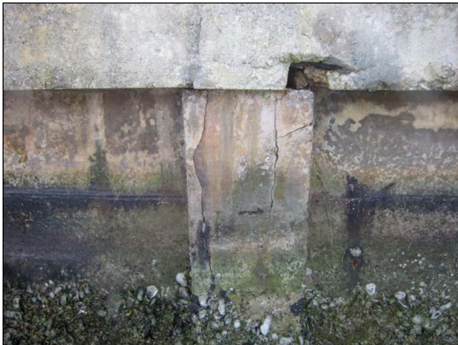
Photo 12: View of a chip in the concrete cap above the T-pile with exposed corroding internal steel. Note cracking, unsound concrete, and rust stains in the T-pile.
