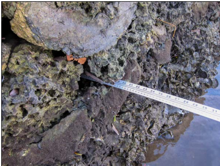
Photo 14: View of 20-inch penetration through a void between separated limestone rocks in the Property bulkhead.
