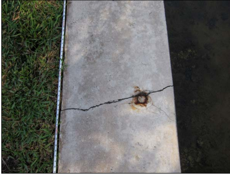
Photo 11: View of an advanced transverse crack in the concrete cap.
