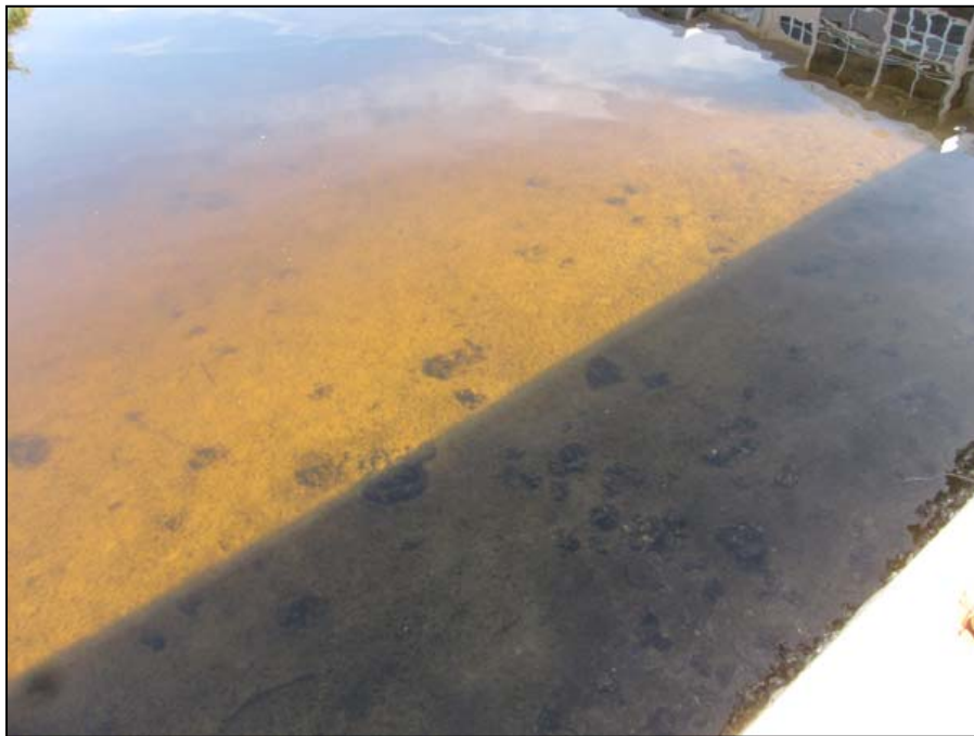
Photo 22: View of accretion of submerged sandy sediment sloping down into the canal immediately waterward of the limestone rock portion of the Property bulkhead.
