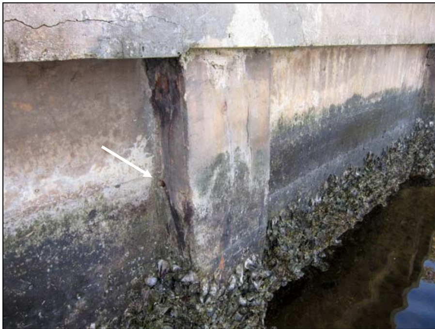
Photo 20: View of a hole within the sealed seam between the T-pile and wall panel.
