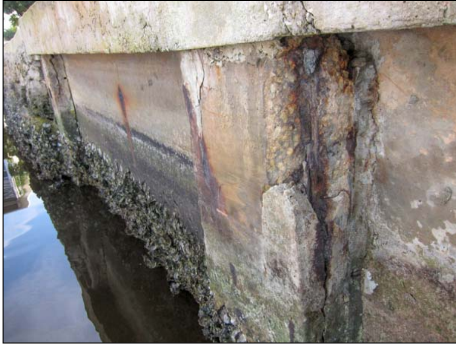
Photo 17: View of typical spalled and unsound concrete with exposed corroding internal steel in a T-pile.
