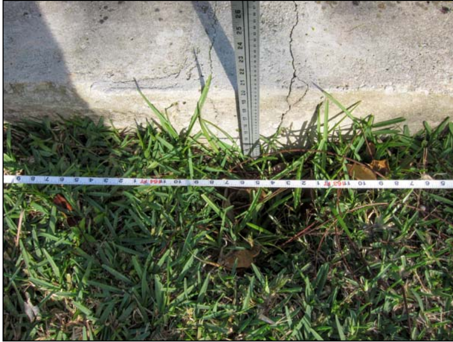
Photo 9: View of a typical depression and erosion in the upland soil with 20 inches of penetration.
