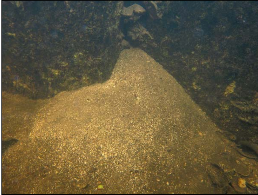
Photo 21: View of typical upland sediment migration through the seam between a wall panel and T-pile at the mudline of the Property bulkhead.
