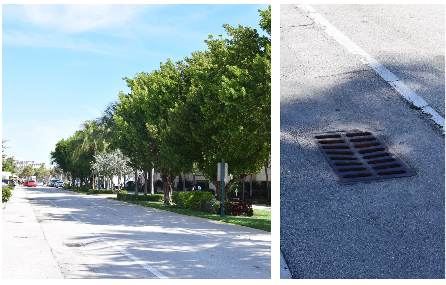
DRAINAGE COULD BE IMPROVED by incorporating retention into the median or along the curb line.
