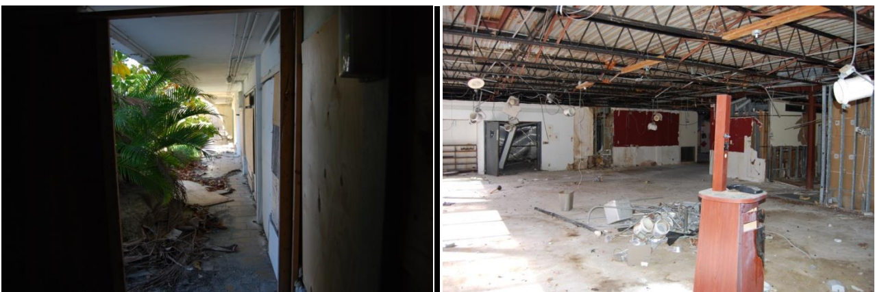
Holiday Inn ground level corridor with debris and plant overgrowth. Denny's interior showing debris.
