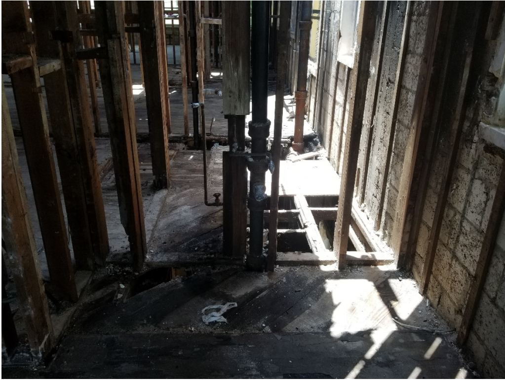
Photo 3 - Hole Burned Through Second Floor
