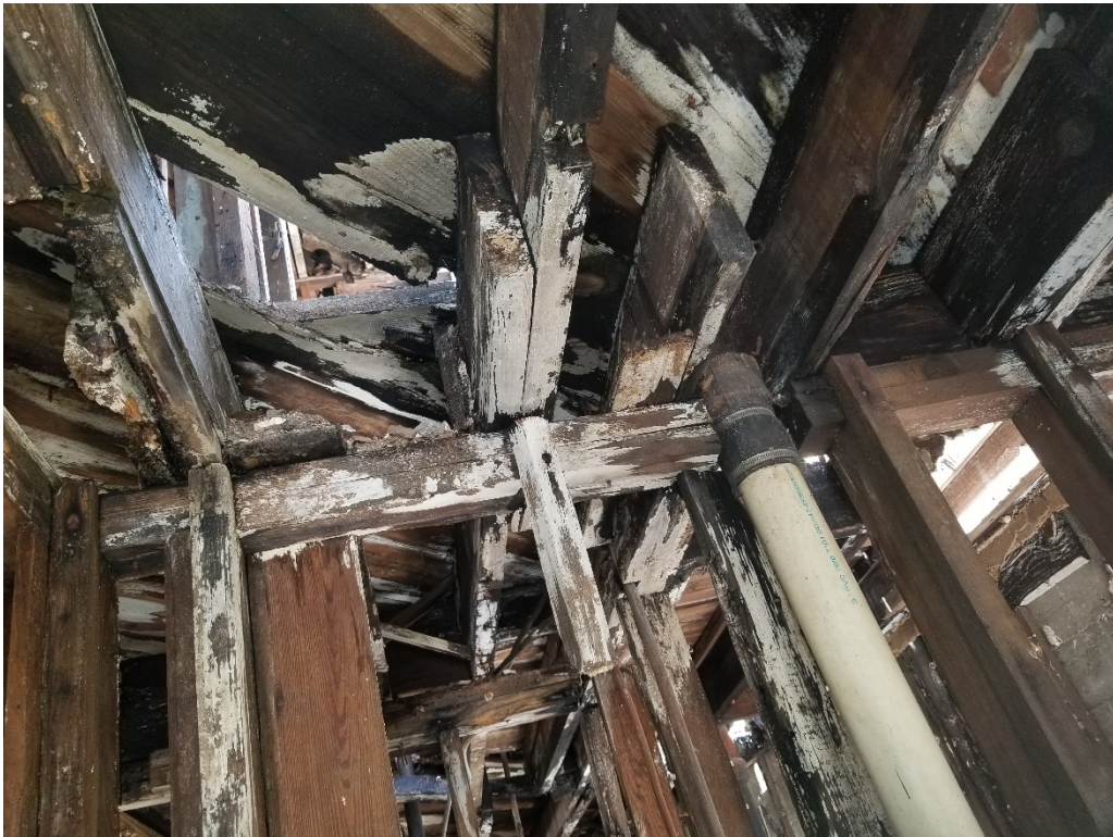
Photo 5 - Deteriorated Second Floor Structure Close up of mold on interior wood structural members.
