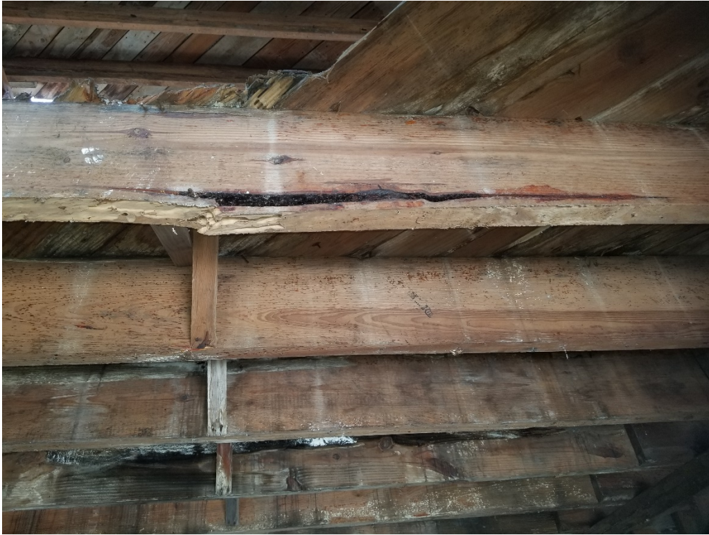
Photo 9 - Termite Damage in Second Floor Joists
