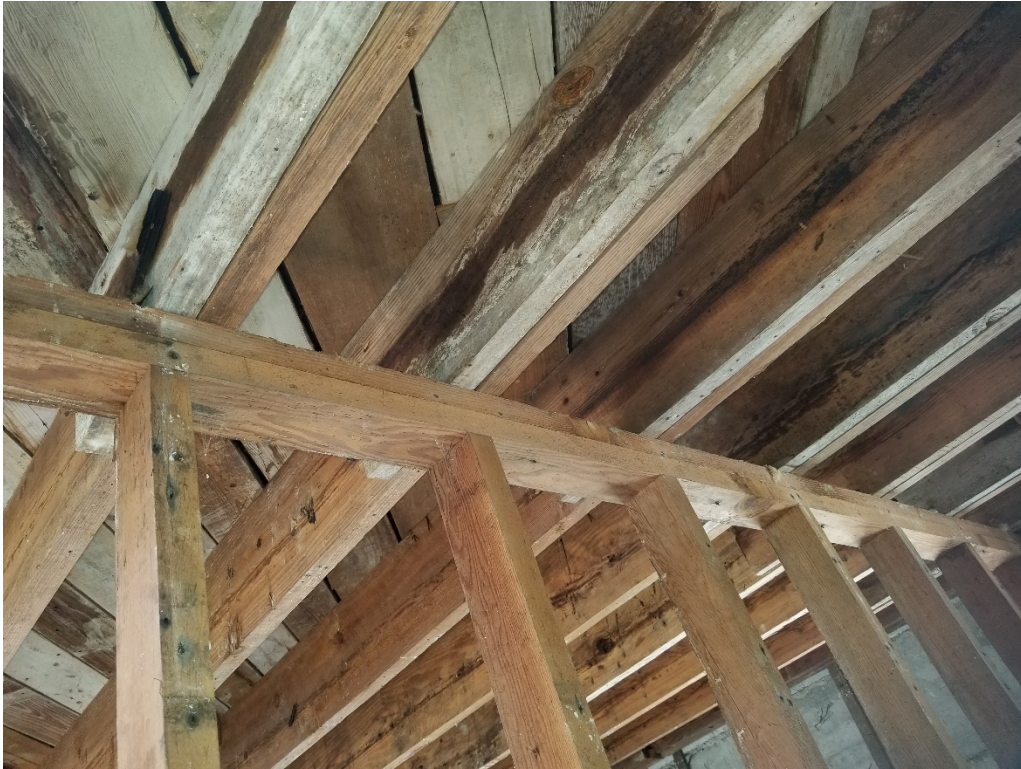
Photo 7- Close Up of Top Plate on Interior Frame Bearing Wall Note that all members are simply toe nailed together. No Simpson style connectors used in the original construction.
