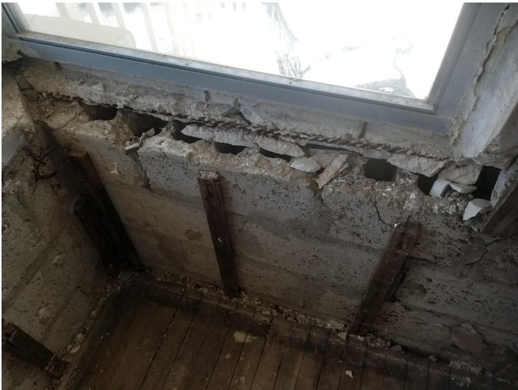
Photo 6 - Spalling Precast Concrete Window Frame Note exposed reinforcing steel due to spalling in precast concrete window frame.
