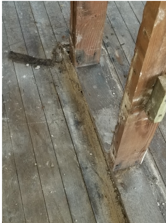
Photo 8 - Close Up of Bottom Plate on Interior Frame Bearing Wall Note that all members are simply toe nailed together. No Simpson style connectors used in the original construction.
