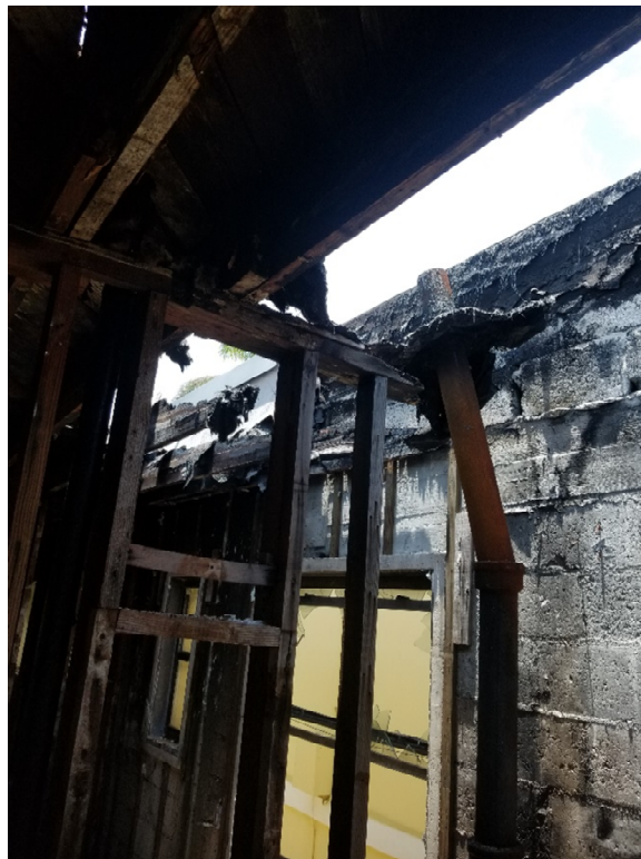
Photo 4 - Hole Burned Through Roof Deck Directly Above Hole in Second Floor
