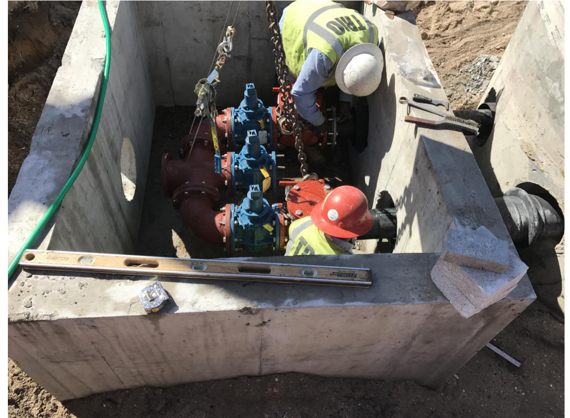
Piping within Valve Vault
