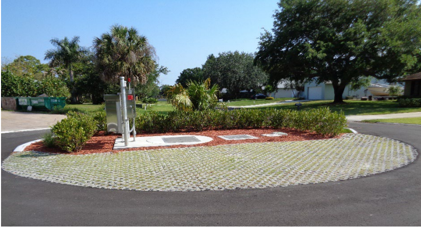
Lift Station Example
