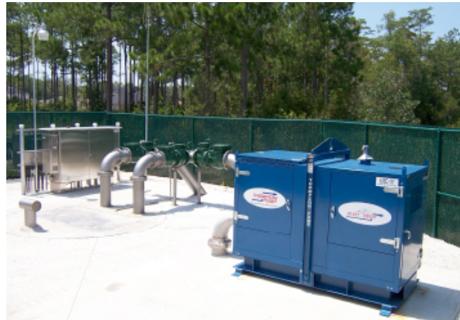
Bypass Pumping Unit
