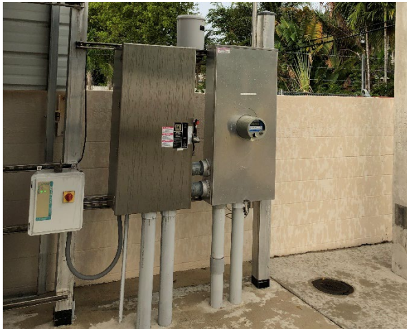
Electric Control Panel
