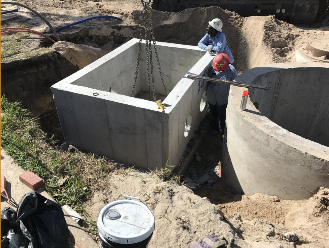
Valve Vault Setting
