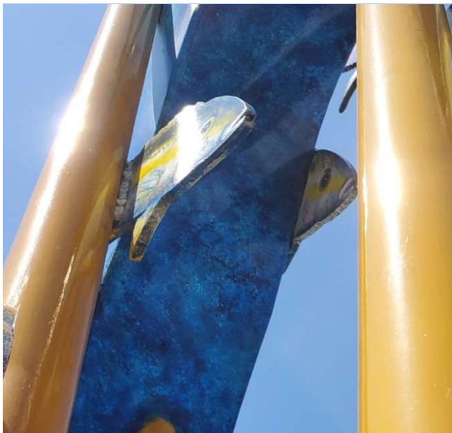
Notice inside of fish's upper mouths and uncoated areas of bare primer on underside of fish tail seen between yellow vertical and blue arch.
