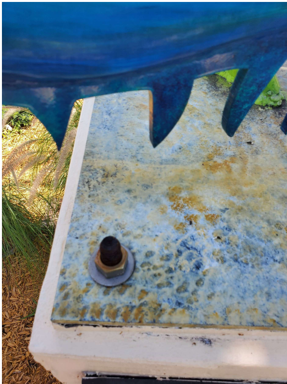
Damage at base attachments
