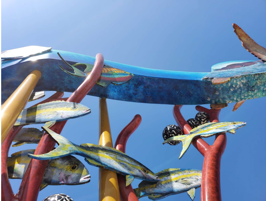
Upward view; notice the black primer visible on underside of upper fin on right side of photo, and visible aluminium and spotting on fin to the left pointing downward. These are examples of what is occurring in different areas throughout the sculpture.
