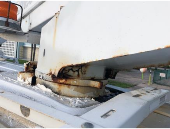
Rust on base of lift and deteriorating roof
