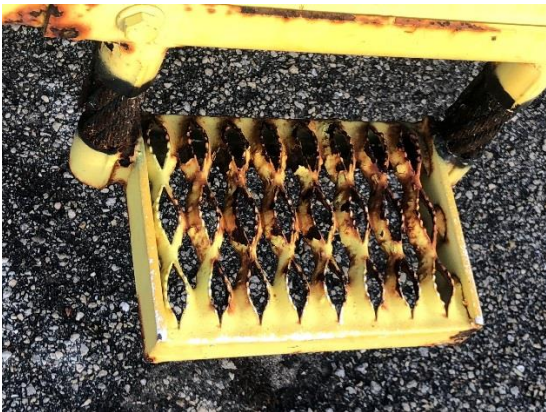
Rusting on step to access the bucket
