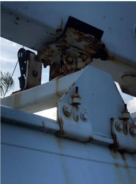
Rust on boom support
