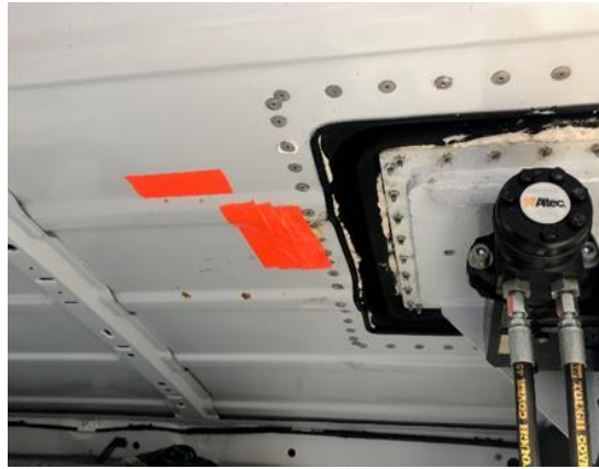
Interior view of deteriorating roof "patch"
