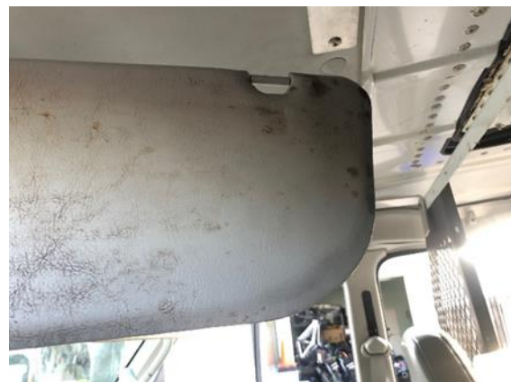
Residual stains from mold
